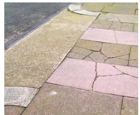
↑ Poorly maintained surfaces can present risks
