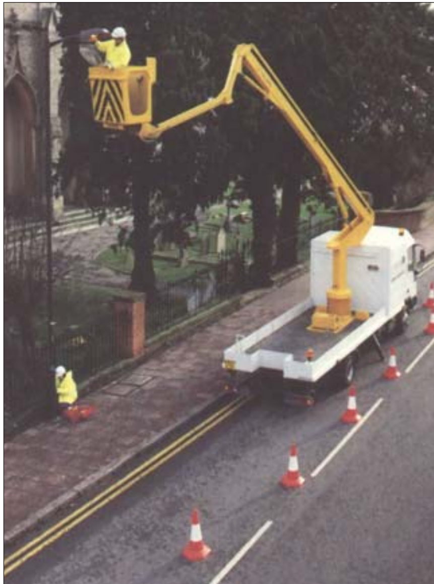
Figure 4.1: Maintenance of 8 m lighting unit. Photograph reproduced by permission of Parkersell Highway Lighting Ltd.
