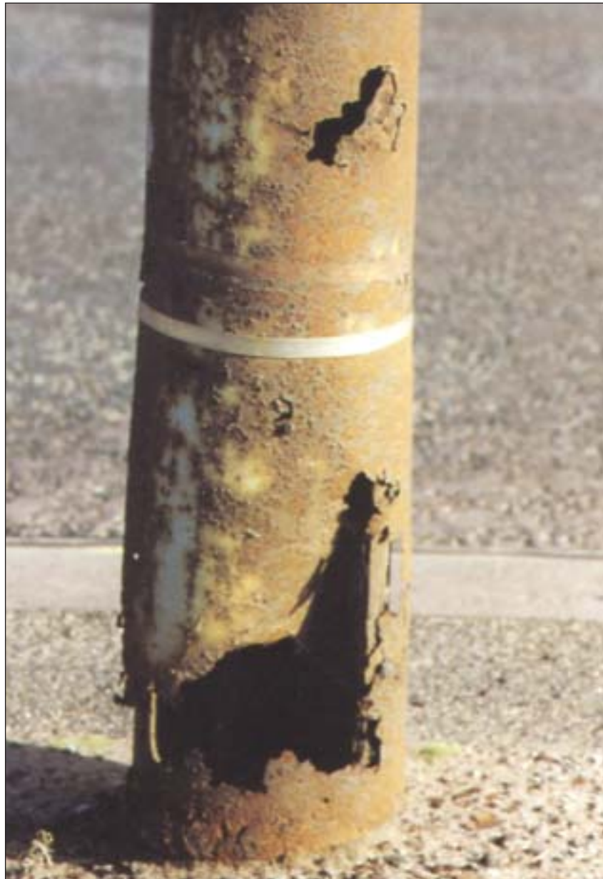
Figure 4.4: Corrosion damage due to lack of maintenance of protective finish
