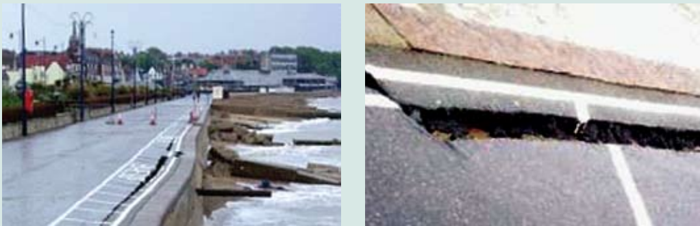
Figure 10.1 Damage to Felixstowe promenade from sea erosion
